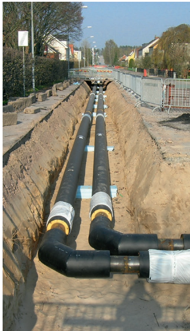
Picture courtesy of Powerpipe
