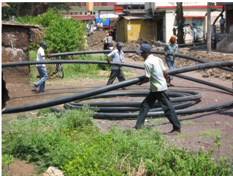
Foto: (c) Borealis India: Improving water infrastructure in Malakpur
