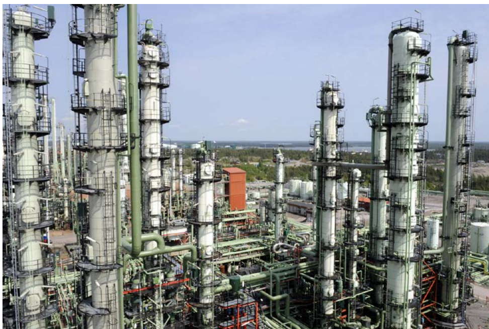
Borealis plant in Porvoo, Finland: phenol and aromatics plant.
