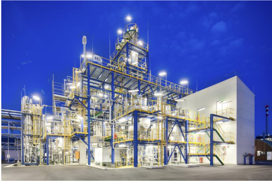
The new Borealis Sirius catalyst plant in Linz, Austria
